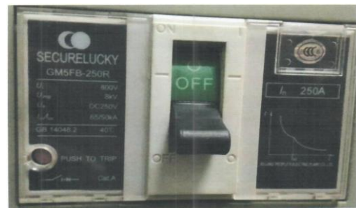
Gambar 8. NFB motor DC oil pump unit 1
