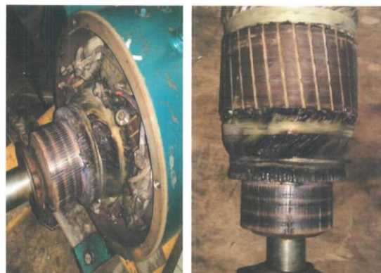
Gambar 6. Kerusakan motor DC oil pump unit 1
